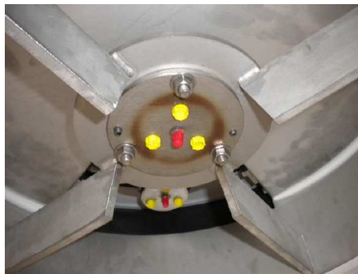
new stainless steel housing bearing arrangement
